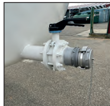
> Vanne raccord pompiers
